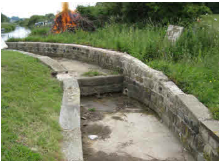
The York Stone copings - missing
