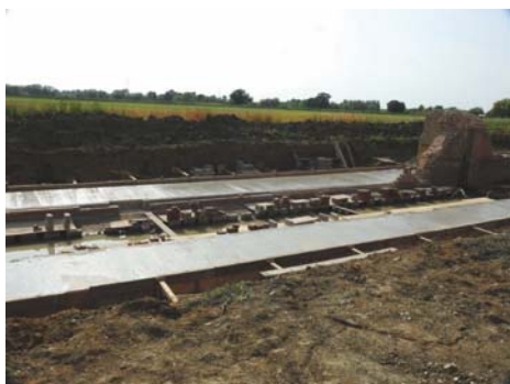
The finished foundations - a brilliant job well done by a stalwart group of volunteers.
